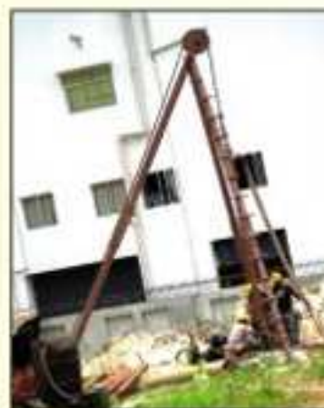
Soil testing for 24x7 water supply project for Dum Dum South Dum Dum and North Dum Dum
