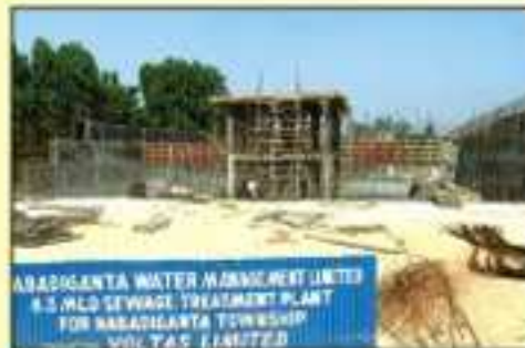
Construction of Sewerage Treatment Plant under sewerage project for Salt Lake Sector-V
