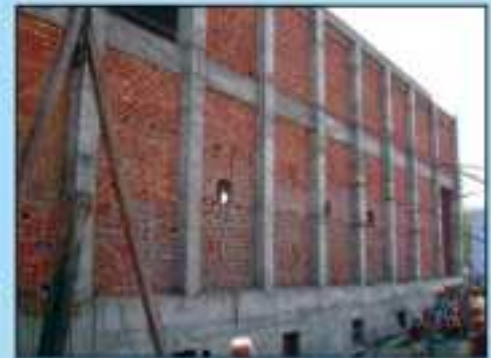
Construction of pumphouse for 3 MGD under ground reservoir and booster station at Gandhi Maidan, Akra
