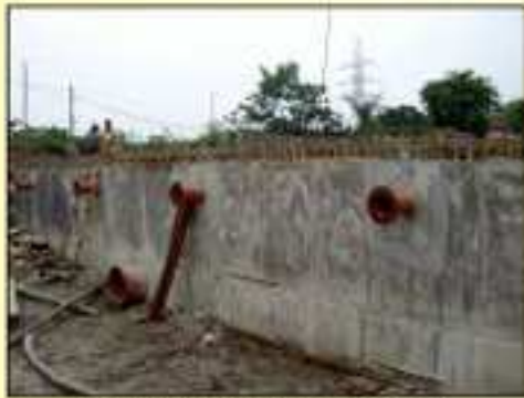
Under Ground Reservoir for water supply to added areas of Howrah Municipal Corporation
