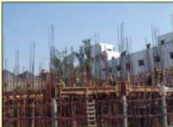
Construction of elevated service reservoir for water supply to Sector-V, Salt Lake
